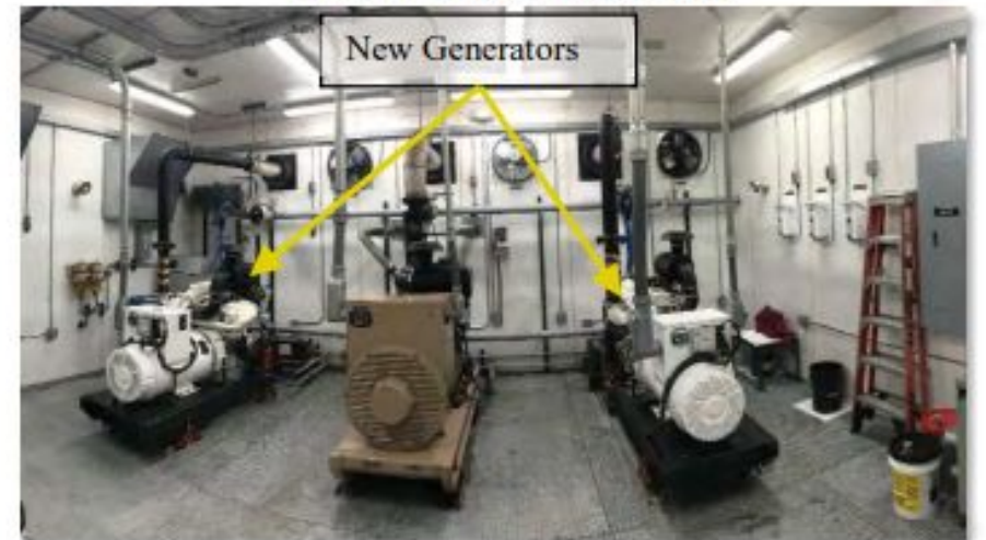
New Tier 3 Diesel Generators
